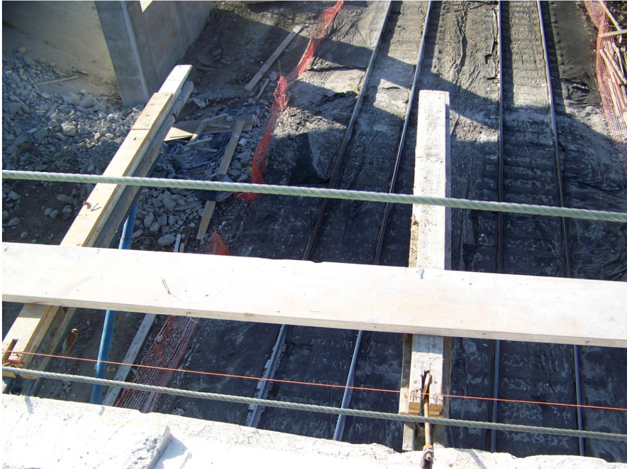
Bridge where worker fell from. Photograph donated by, and property of, Kentucky State Government.
